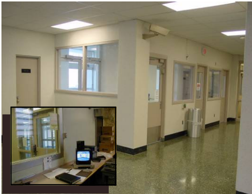
Above: Access Control & CCTV Monitoring
