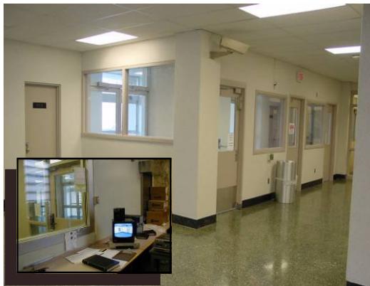
Above: Access Control & CCTV Monitoring
