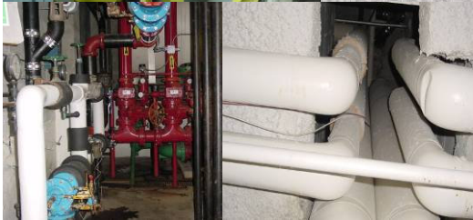
Above: Utilizing Existing Systems allowed for cost-savings to the owner
