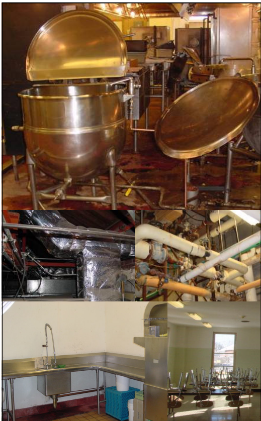
Above: Every major system was in need of updating.
