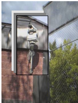
Right: The perimeter is secured by both security fencing and CCTV Monitoring
